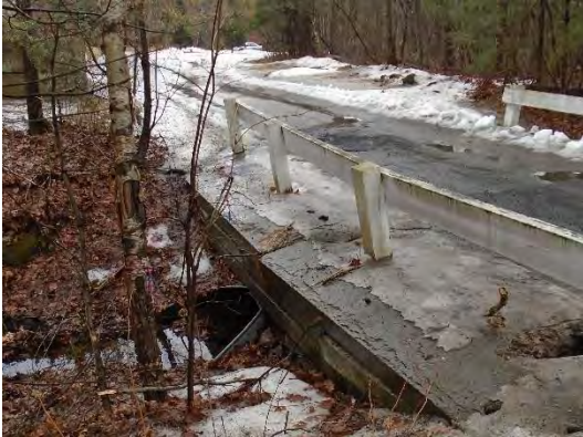
Representative settlement headwall failure.
