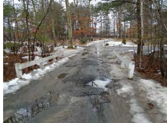
Road surface condition over the culverted crossing.
