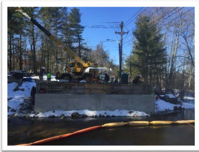
Pouring the Concrete for the West Abutment Backwall and Wingwall Caps - Looking West
