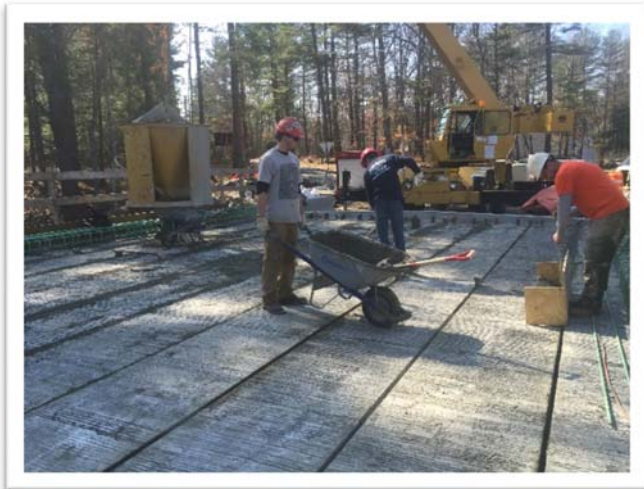
Pouring the Grout on the Shear Keys Between the Concrete Beams - Looking West
