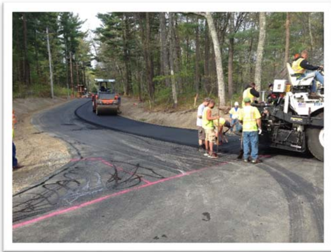
Paving Wearing Course at Town Farm Road – Looking South from Bluff St Extension
