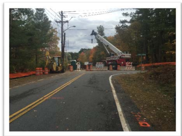
Cofferdam Installation at New West Abutment Location Looking East from Bluff St Ext
