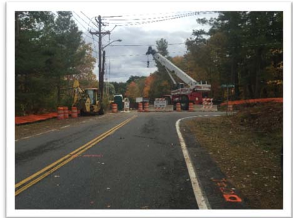
Bridge Closure Looking East from Bluff St Ext
