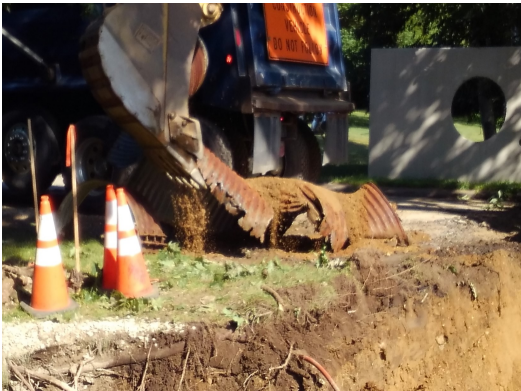
Rusted old pipe....
