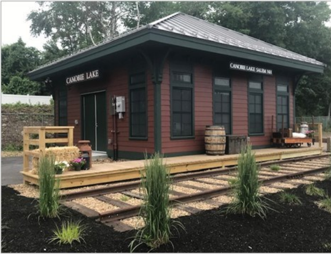
Regional Water Line PRV Station at the Rail Trail Parking by Windham town line. It was designed to replicate the Canobie Lake Railroad Station that once stood near this location.
